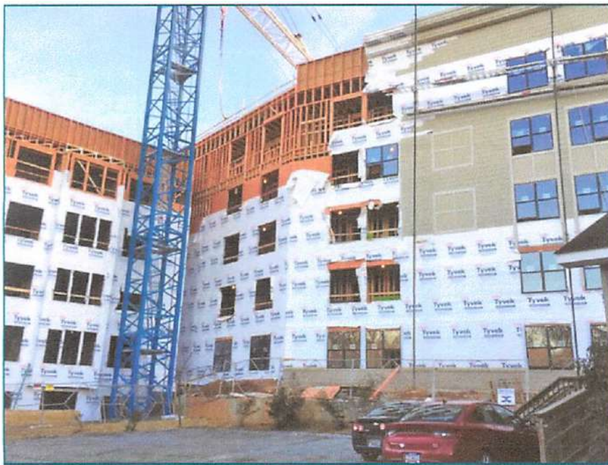
Figure 11 – A haphazard sequencing of multiple trades on the exterior wall of a building under construction.
