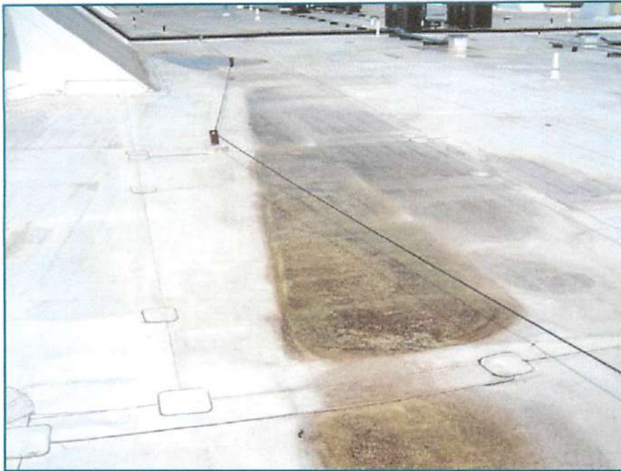
Figure 2 – Typical ponding where the valley of a roof cricket is less than ¼ inch per foot.
