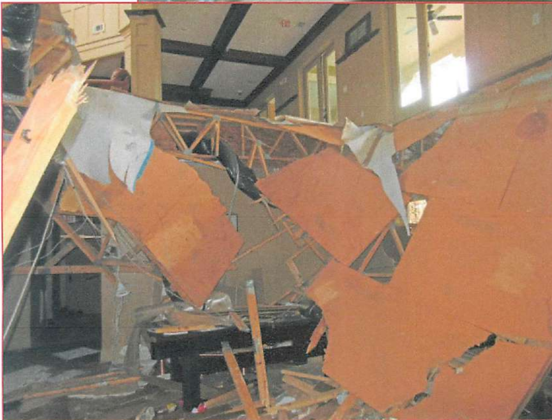
Figure 3 – View of collapsed floor framing.
