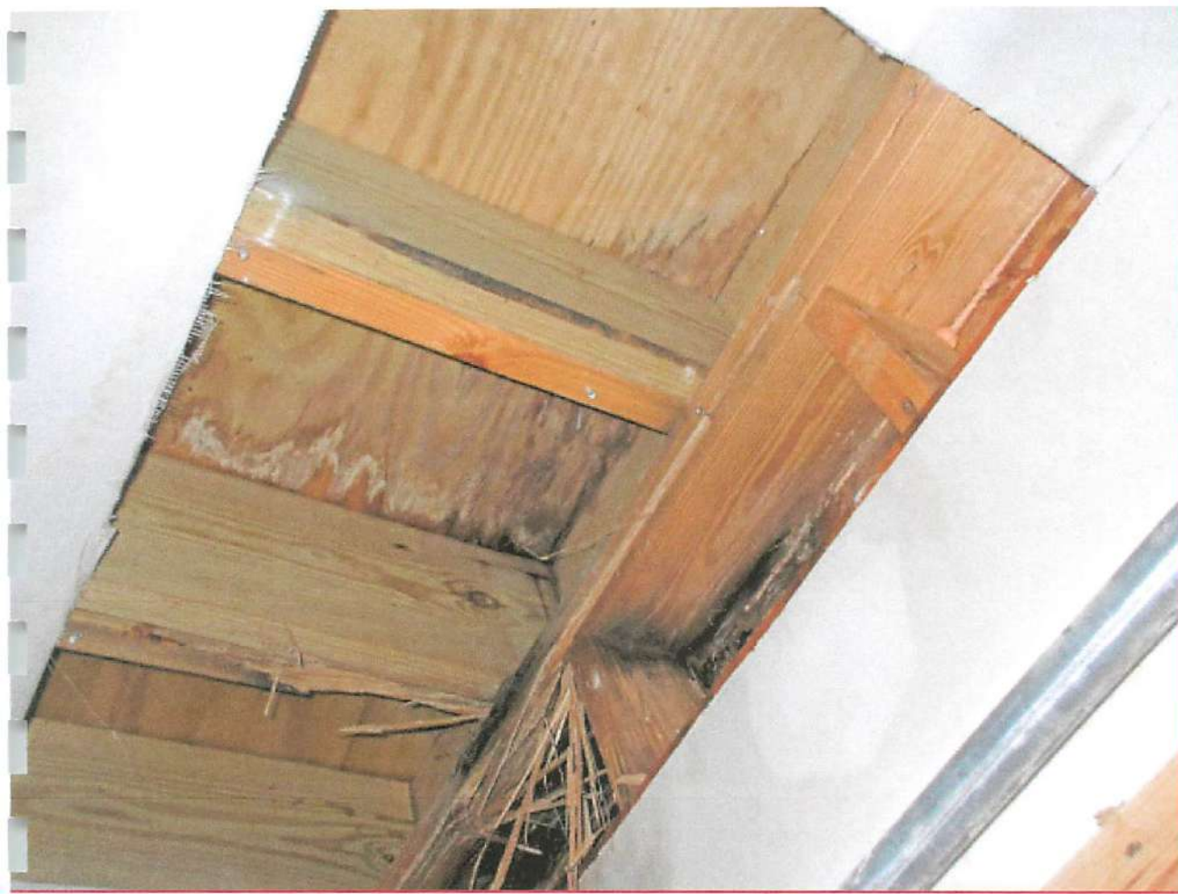
Figure 6 – View of water damage at balcony.
