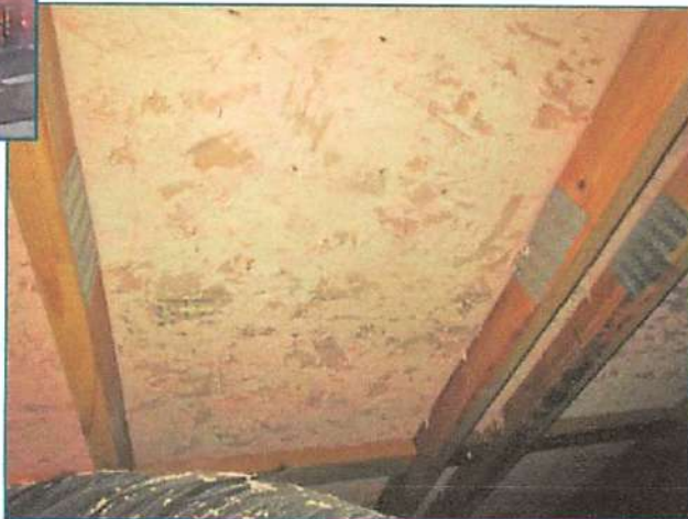
Figure 4 – Failure of fire-resistant paint that was intended to protect a combustible OSB roof deck.
