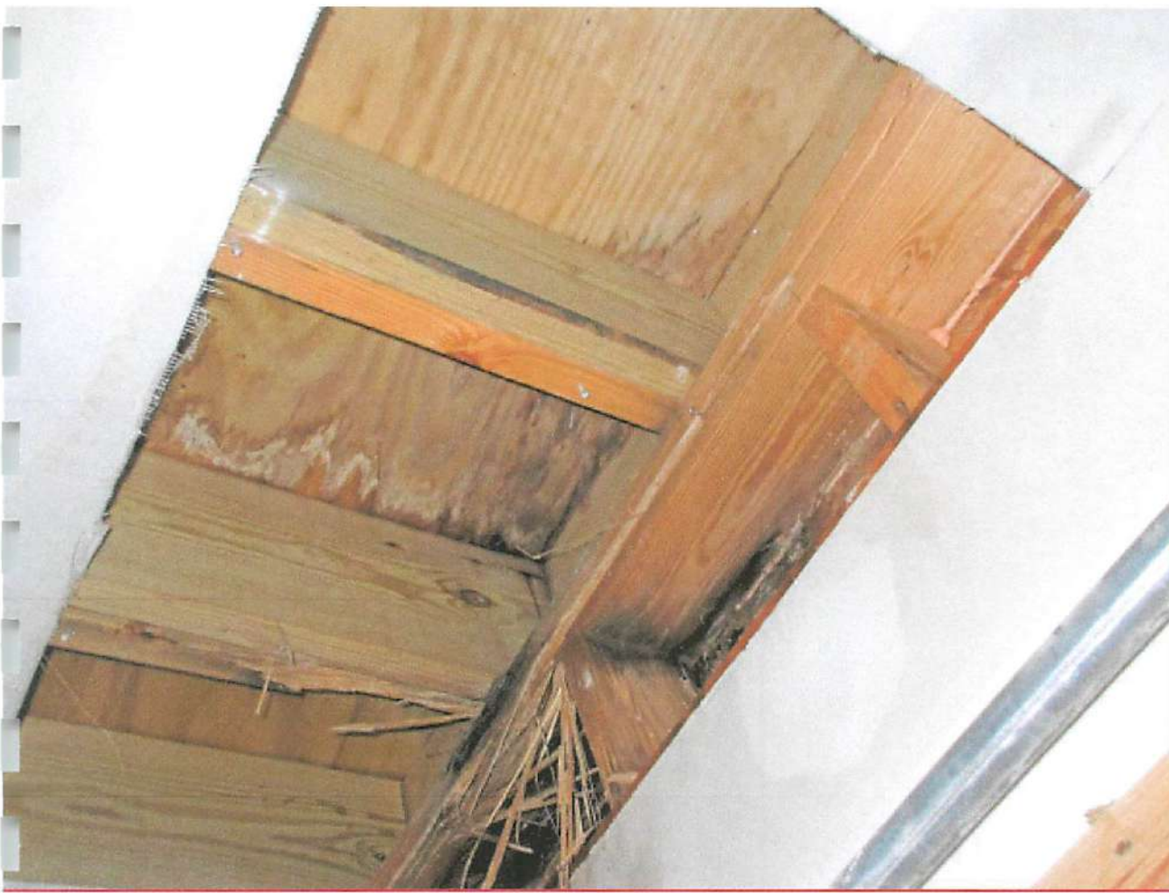
Figure 6 - View of water damage at balcony.
