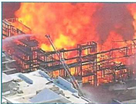
Figure 3 – Mid-rise wood-frame building fire in Kansas City, Kansas.
