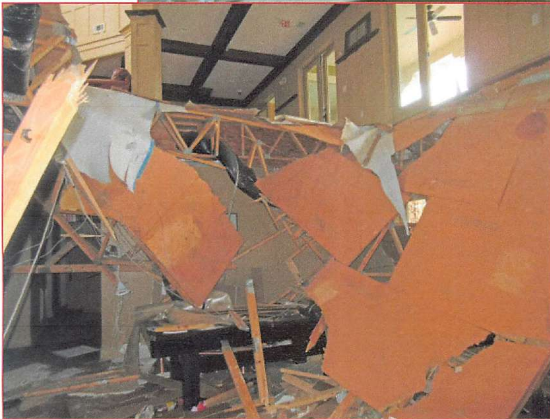
Figure 3 – View of collapsed floor framing.
