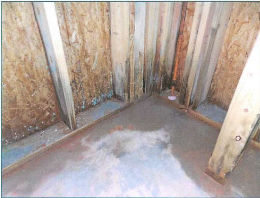
Figure 10 - Water intrusion/damage of a mid-rise wood-frame building under construction.
