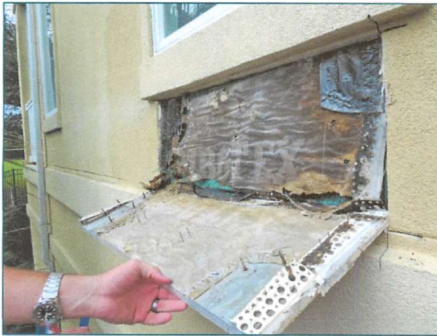
Figure 8 - Moisture damage behind stucco caused by improper integration of two layers of WRB.
