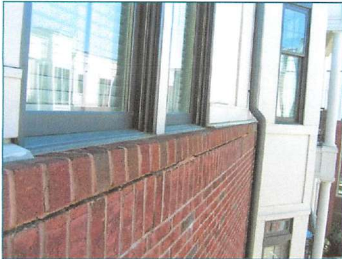
Figure 7 – Brick damage caused by differential building movement.
