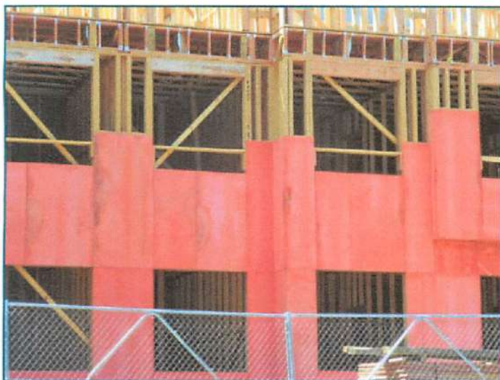
Figure 5 – Water-damaged fire-resistant paint that was intended to protect combustible OSB wall sheathing.
